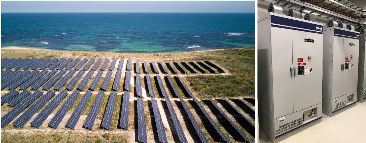
Garden Island Microgrid's solar array and battery energy storage system
