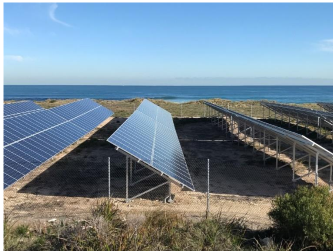
Garden Island Microgrid
