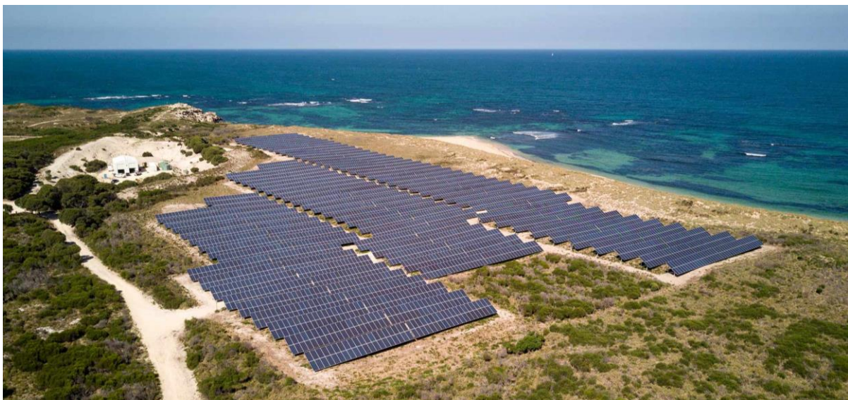
Carnegie's Garden Island solar array
